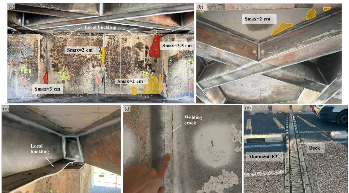
Figure 1. Post-fire visual inspection of the “Bridge of the Flowers”. (a) Overall view of the most damaged area indicating maximum spalling ( S_{max} ) in Abutment 2 as well as the diaphragm girder main damage. (b) Concrete deck spalling and overall view of out-of-plane displacements. (c) Detail of local buckling on diaphragm girder. (d) Detail of welding crack, (e) Detail of deck uplift movement noticed by the inclination of the expansion joint
