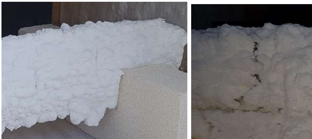
Figure 14. Foam drips and cracks
