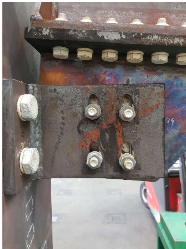
Figure 10. Deformation of the connection after the test (after cooling)
