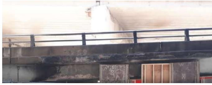
Figure 5. Post-fire photo of an overpass in August 2020 with fire occurring in March of 2020 (Author's photos)
