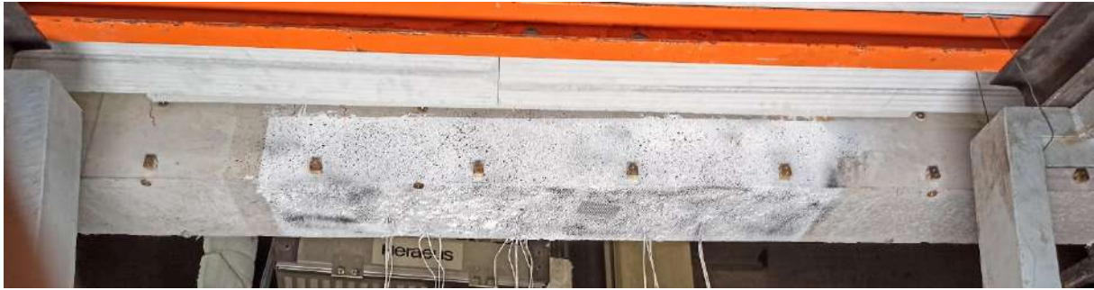
Figure 4. The compressed side of the beams monitored using the Digital Image Correlation (DIC)
