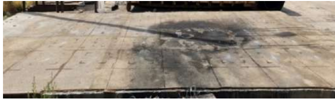
Figure 6. Post-fire surface of the slab
