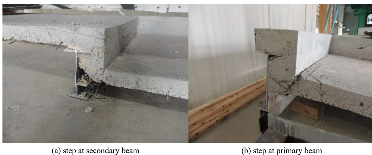
Figure 14. cracks at the step
