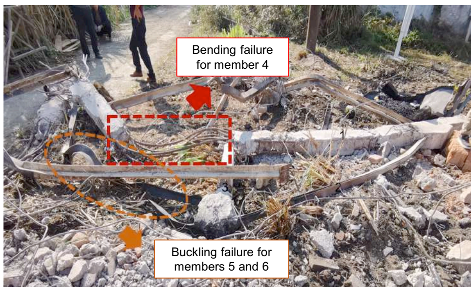
Figure 6. Collapse mode of the truss
