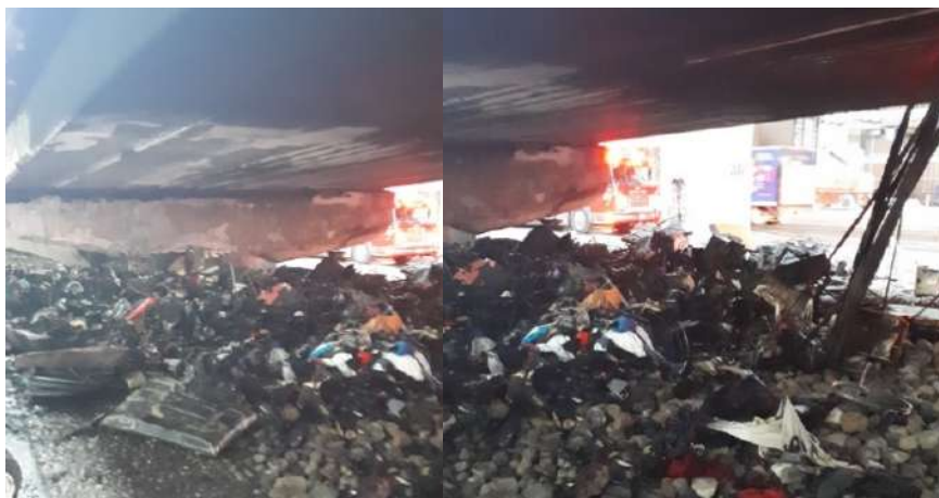
Figure 4. Post-fire photo of an expressway in February 2020 (Author's photos)
