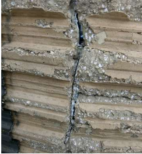
Figure 21. Failures of the welded wire mesh
