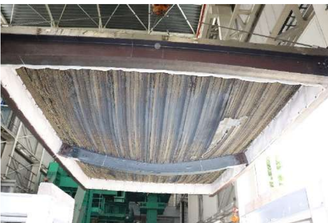
Figure 19. Damage to the exposed surface
