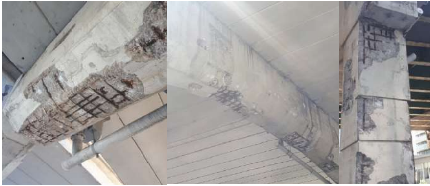
Figure 2. Corroded concrete beams and columns on an expressway in 2020 (Author's photos)
