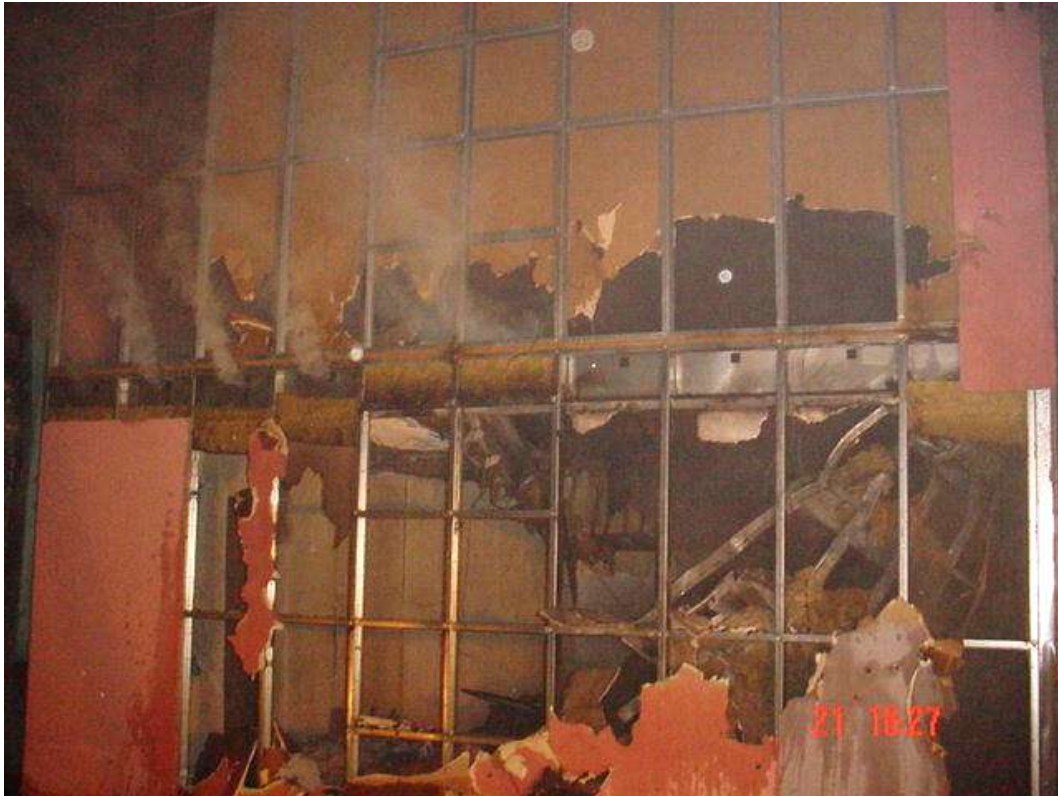
Figure 2. Collapse of floor slab in latter stages of fire experiment
