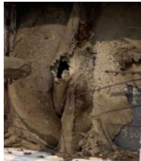
Figure 3. Impact of jet fires on fire protection
