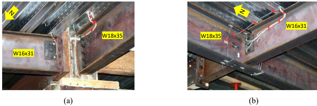
Figure 2. (a) Beam- and girder-to-column and (b) beam-to-girder single-plate shear connections in the CF2 Test [4] (W-shapes in U.S. customary units)
