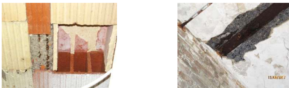
a) defects present to the underside of a hollow pot floor system b) defects present to the underside of a filler joist floor system
