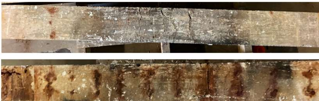
Figure 10. Visual impact of corrosion to 60 MPa beams at 10% mass loss (top) and 30% mass loss (bottom)
