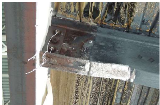
Figure 20. Damage of the bolted connection
